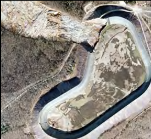
Orthoimagery of failed Taum Sauk Reservoir
